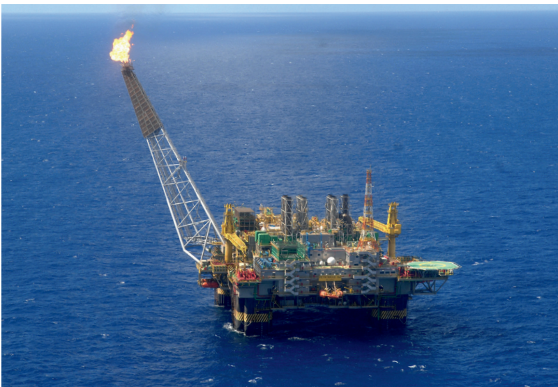
Fire water pumps on P52 FPU. Photo: Courtesy of Petrobras.
