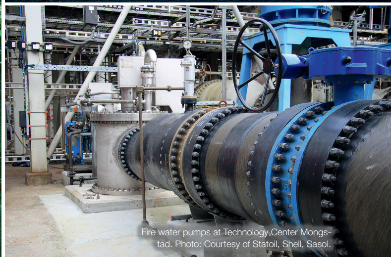
Fire water pumps at Melkøya gas terminal. Photo: Courtesy of Statoil.
