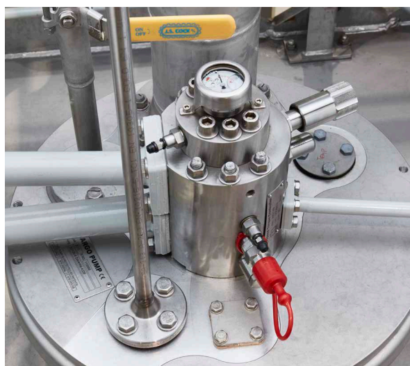
STC valve on cargo pump top
